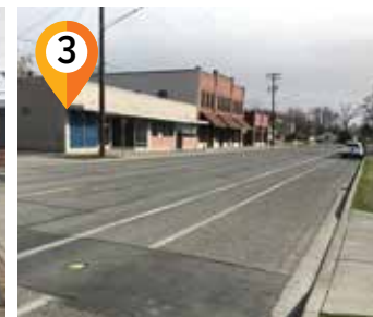
3 2nd Avenue Pavement Preservation Replacing existing asphalt surface, utility adjustments, and re-striping; from Birch to Howard
