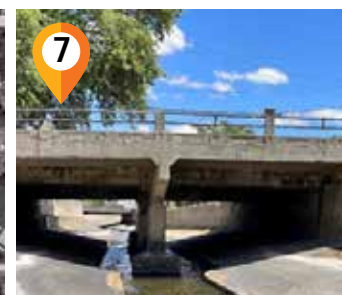
7 5th Avenue Bridge Replace the existing bridge over Mill Creek with a bicycle and pedestrian bridge
