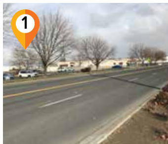
1 Rose Street Pavement Preservation Crack sealing, chip and fog seal, re-striping, and signal upgrades; from College Place to Isaacs Avenue
