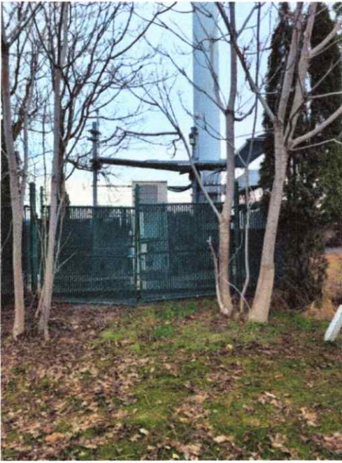
See Above: Cell Tower located at The Municipal Golf Course. This tower has a gas meter. The Cell Tower at 928 Sturm Avenue will look similar but have a 450-gallon diesel tank next to a stream.
