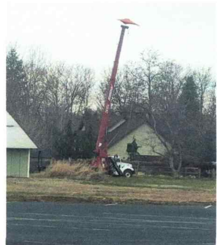
See Above: 1131 East Chestnut. View from side of home. Cell tower will be only 65' from fence. Antenna arrays will come down to top of home's roof. This is also the view from Lot 10 and 11 at Bryant Park Subdivision. These 2 story homes will have upstairs views of the 65' tower and look down onto the equipment base. Trees will never grow tall enough to screen the cell tower. All homes at Bryant Park Subdivision will have a view of the cell tower.
