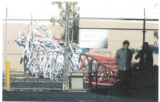
Cell tower collapses during construction.
