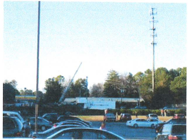
Welding causes cell tower fire near daycare center. Lilburn, GA, Dec 1, 2011 https://www.gwinnettdaily.com/archive/cell-tower-fire-closes-rockbridge-road-evacuates-day-care/article_c799bdd9-1162-52a6-8cd7-
