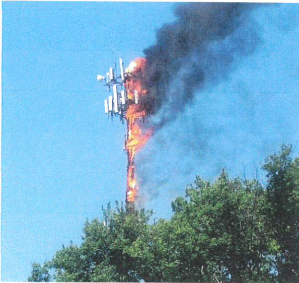
Cell tower fire caused by improper welding. Bensalem, PA, June 21, 2013
