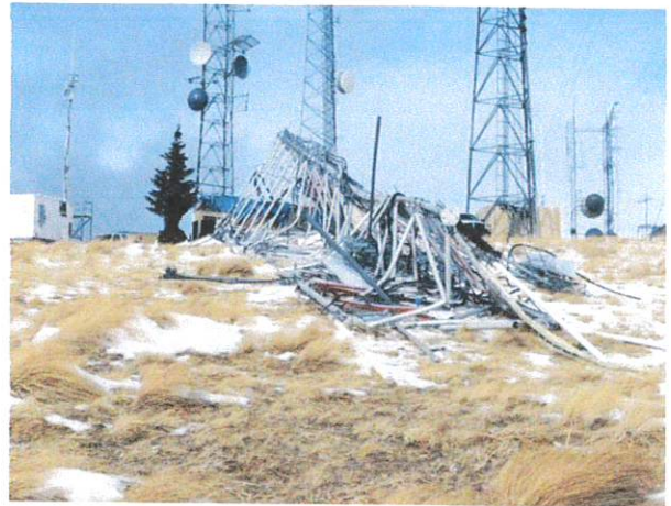
Cell tower collapses in high winds.
