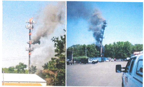
Welding causes cell tower fire. Bensalem, Pa, June 21, 2013 http://levittownnow.com/2013/06/21/nearby-cell-tower-on-fire-may-collapse/ Photo credit: Twitter.com/Mz_Erica7801
