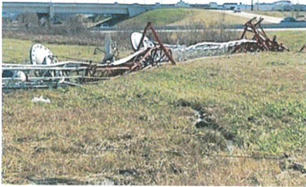
Cell tower collapse in high winds. Broken Arrow, OK, Dec 9, 2009
