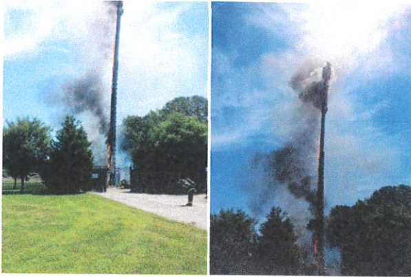
Cell tower fire caused by improper welding near Heritage High School. Newport News, VA, Jun 16, 2015 http://wtkr.com/2015/06/16/cell-phone-tower-near-heritage-high-school-catches-fire/ Source: WTKR3
