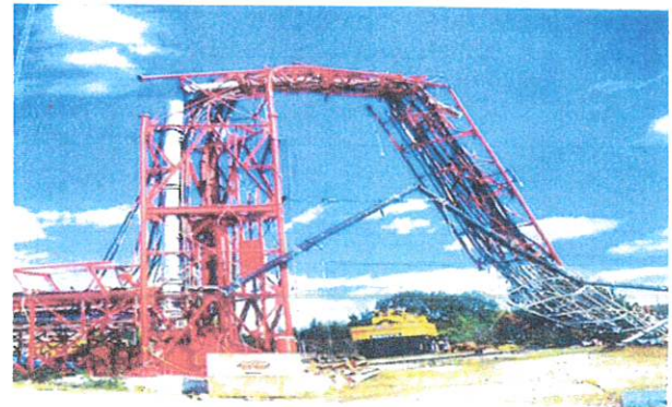
Cell tower collapses during maintenance, killing three workers.
