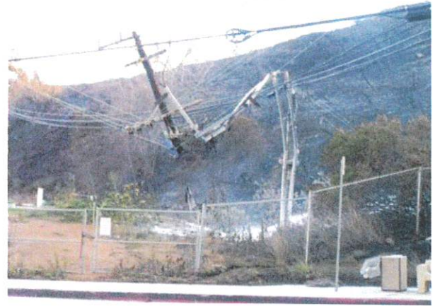
Malibu Canyon fire, 2007 Overburdened with weighty telecom gear, the pole collapsed. 14 houses burned.
