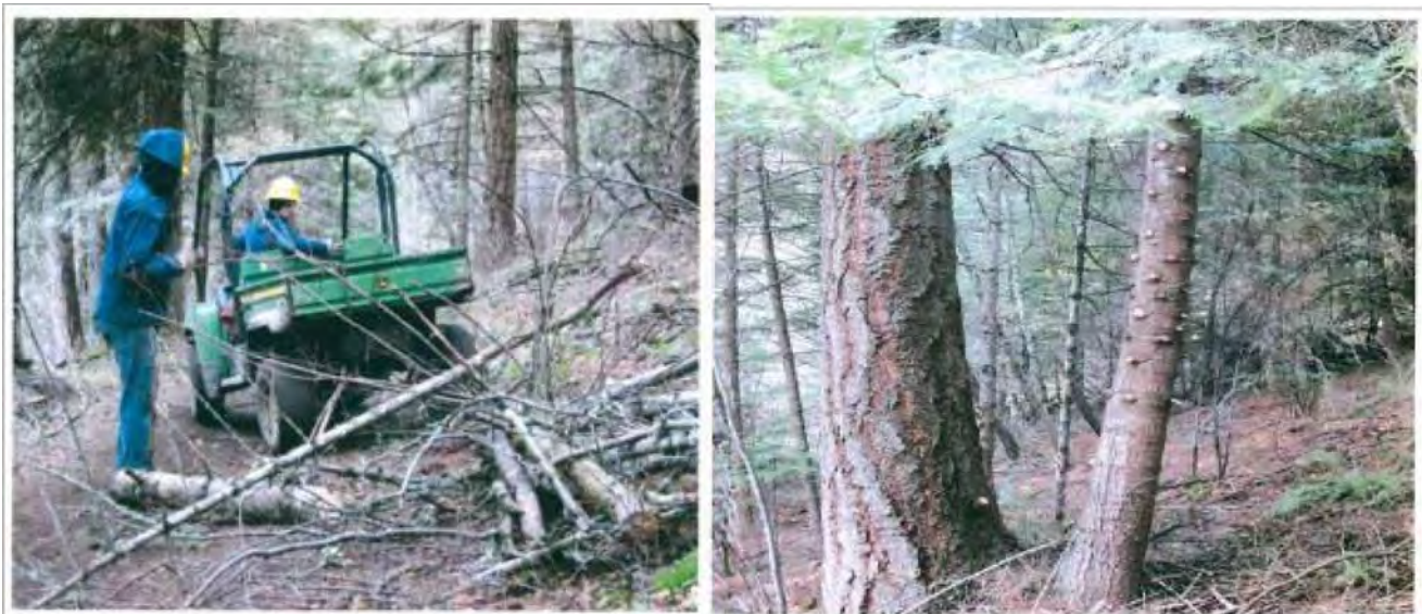
Figure 21 City of Walla Walla fuel reduction projects within their properties along Mill Creek and their intake facility
