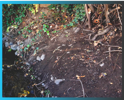
Area prone to erosion
