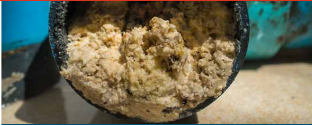
This is a drain pipe with a big FOG clog. Not only is it gross, it reduces the diameter of your pipe and can create blockage.
