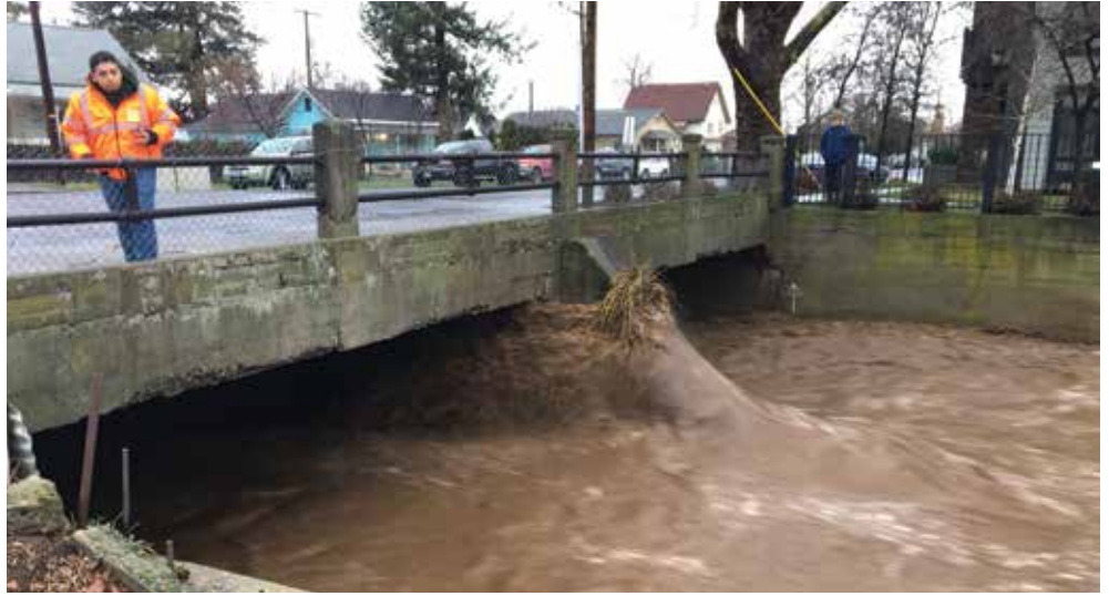
During the high-water event on Feb. 7, City employees from Public Works and Parks & Recreation monitored the condition of the Mill Creek bridges and levees to help ensure the safety of residents.
