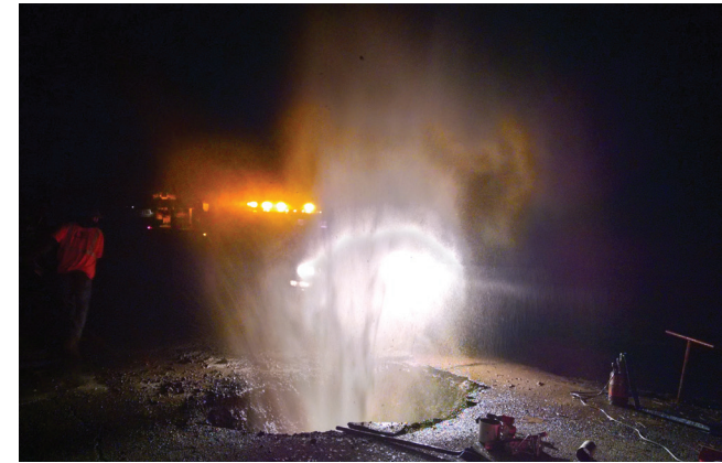
City workers fixed this leak on Middle Waitsburg Road, which was losing an estimated 200 gallons per minute.
