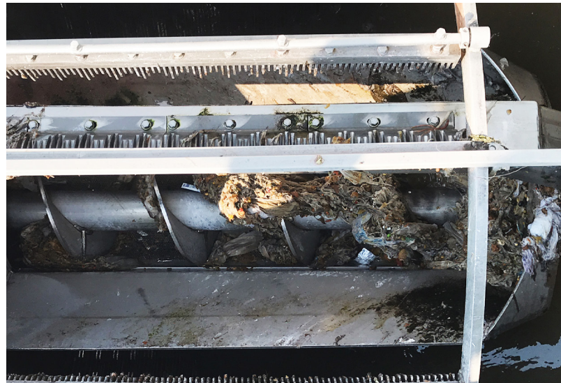
Above: Screens at the Wastewater Treatment Plant catch paper and other insoluble material.
