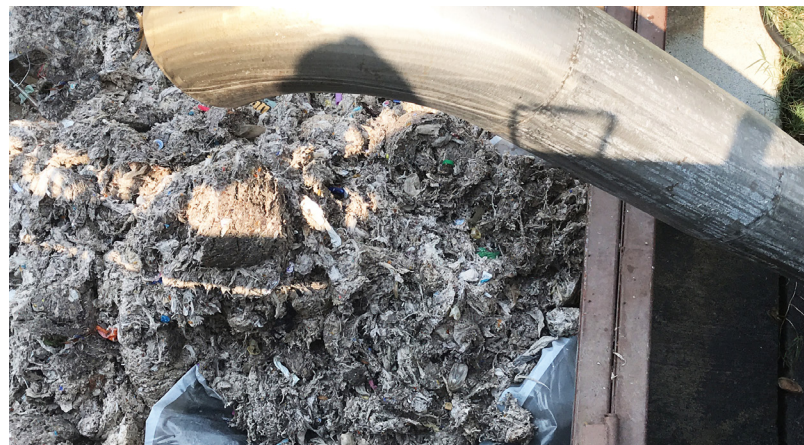
Below: An auger pushes the material up a pipe into this bin. “Flushable” wipes and other paper hygiene products compose half of the material that we dispose of at the plant.
