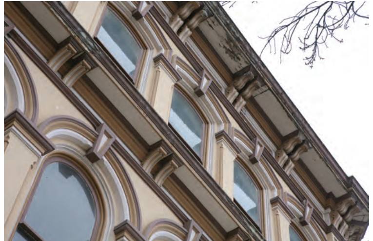
2017 view looking at the cornice and bracket details on the building at 2 E Main Street. Courtesy Artifacts Consulting, Inc.
