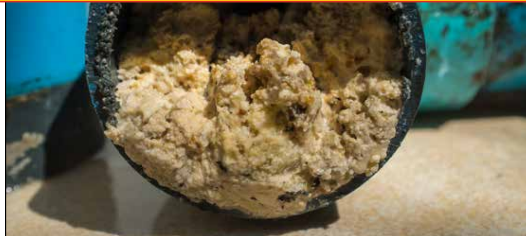
This is a drain pipe with a big FOG clog. Not only is it gross, it reduces the diameter of your pipe and can create blockage.
